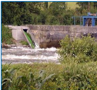
Crawling gutter fixed on a manhole at the end of the upstream by-pass channel.
